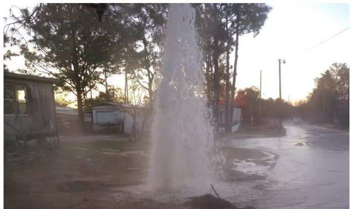
This broken main water valve at ROI Strategies’ mobile home park was easily fixed, but it’s a good reminder of why it’s better to be an investor and not a landlord!
